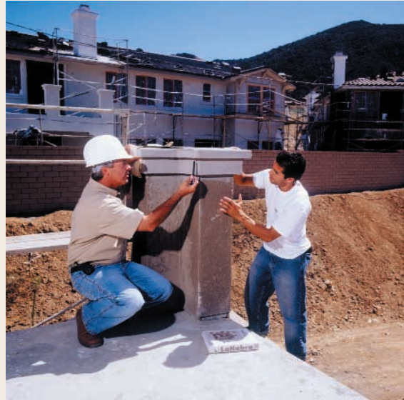
From the time product leaves the plant until the project is completed, LaHabra Stucco is your partner on the job.
